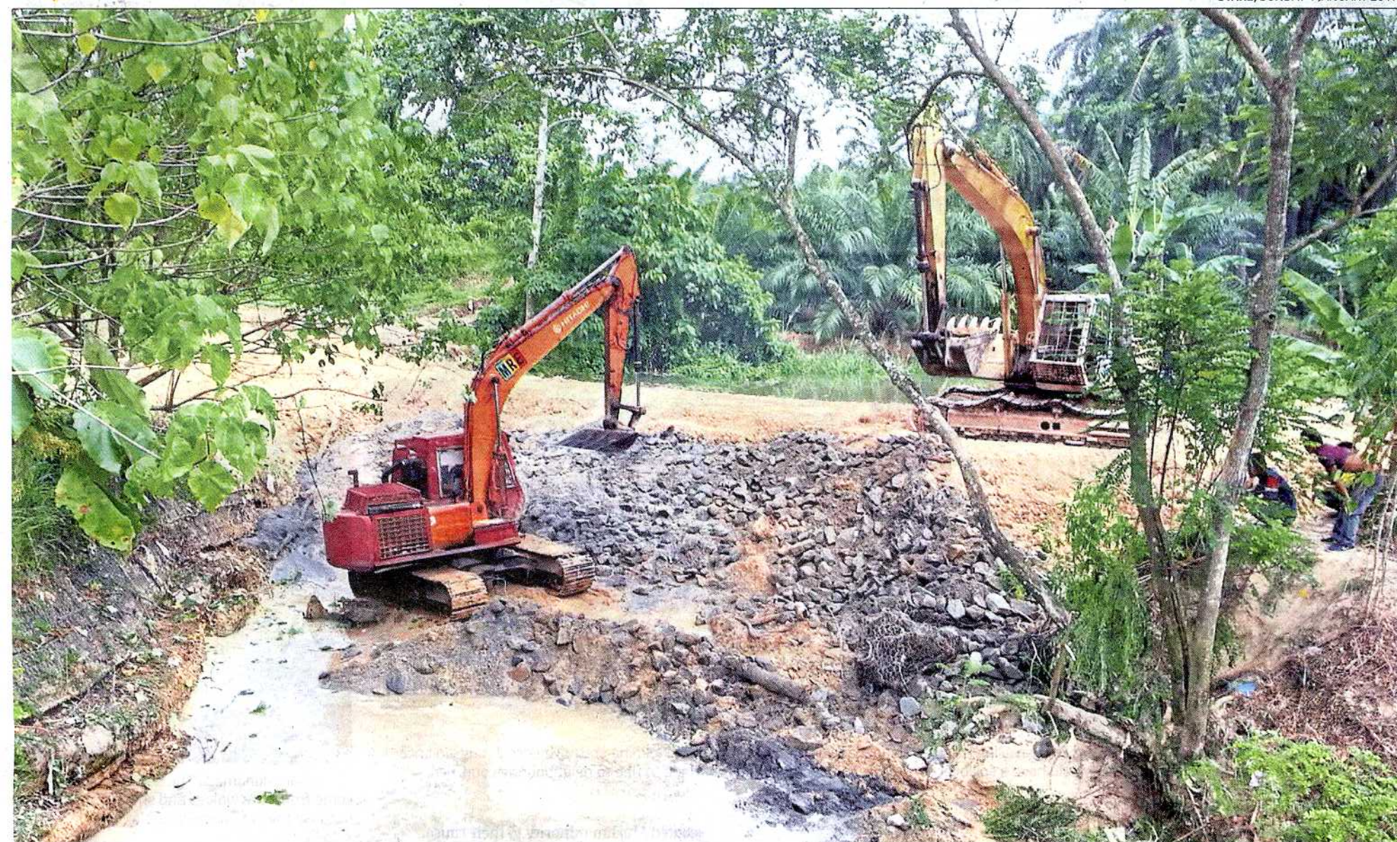
Water woes: Air Selangor workers using excavators to block the flow of water from the contaminated Sungai Buah into Sungai Semenyih last October. It took authorities a while to identify the contaminant in this incident, underlining the need for more advanced treatment technology that can deal with emerging pollutants. — Photos: Filepics
