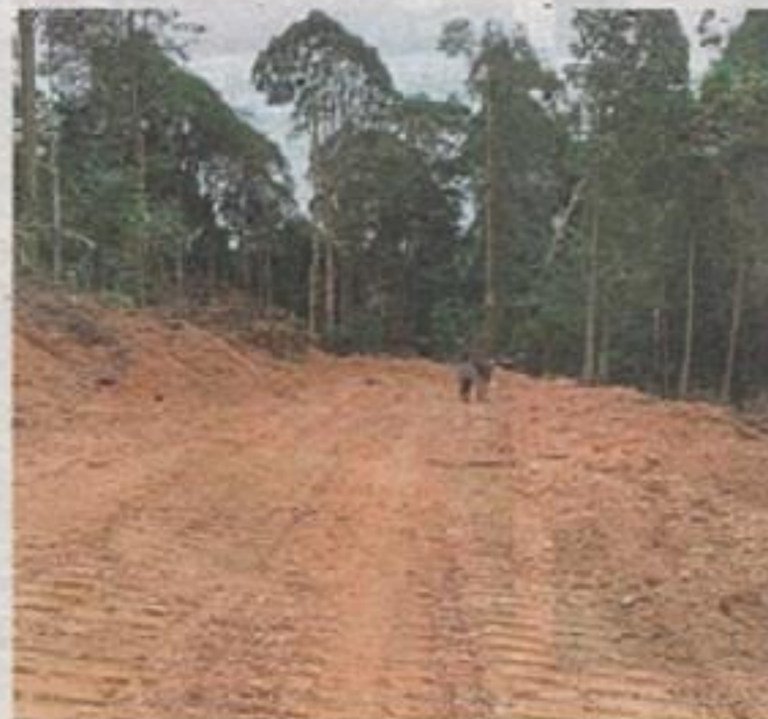
Land clearing works going on at a portion of the land in Bukit Cerakah for a residential project, which has been approved by the authorities.
