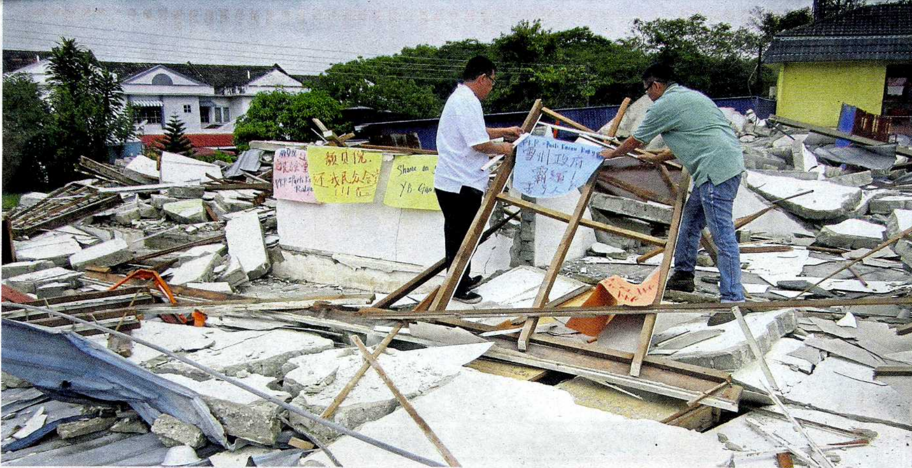
Selayang MCA members going through the debris at the site of the demolished MCA community hall in Taman Bukit Rawang.
